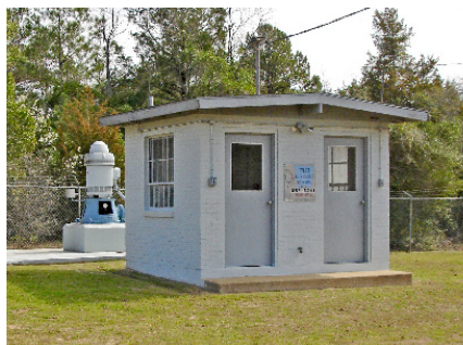
Tyler Water Utilities well on Robertson Road
