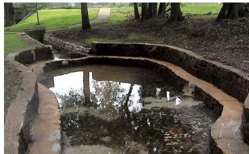
The City should seek education on preservation of its historic infrastructure, including City Park Spring Pond, a Tyler Historic Landmark on West Queen Street.
