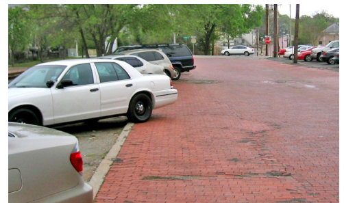
Historic brick streets require special maintenance.
